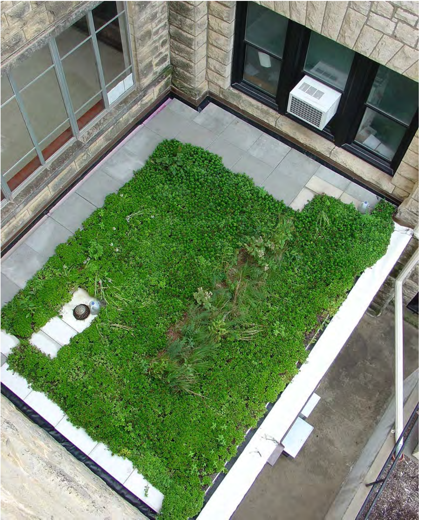
Photo by Lee R. Skabelund – August 5, 2013 amid the second full growing season on the lower green roof. Note that supplemental irrigation (by hand-held hose) is being provided on an “as need” basis (in other words, when soils are dry and vegetation is stressed).
