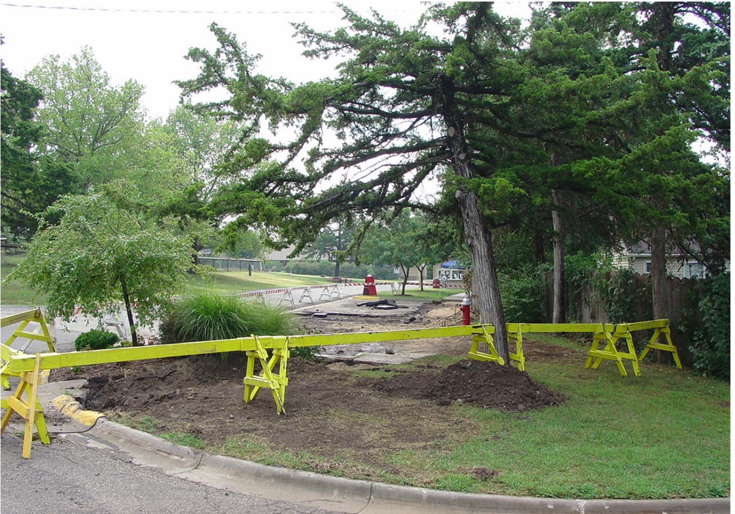
Photo by Lee Skabelund – August 30, 2011 during tear-out of impervious asphalt and concrete paving.
